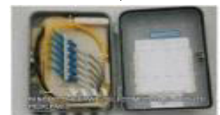
Building distribution box
