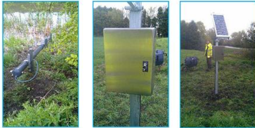
Fig. 3.7 Xylem Solar Pumps
